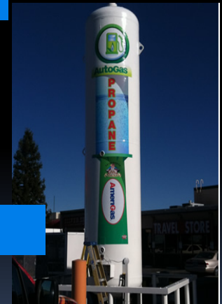
Vertical 1,990 Gal Dispenser Station
