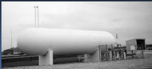
30,000 Gal Bulk Storage Facility (transport delivery)
